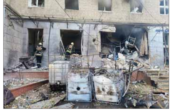
Rescuers inspecting a damaged hospital building following a drone attack in Sumy. (AFP)
