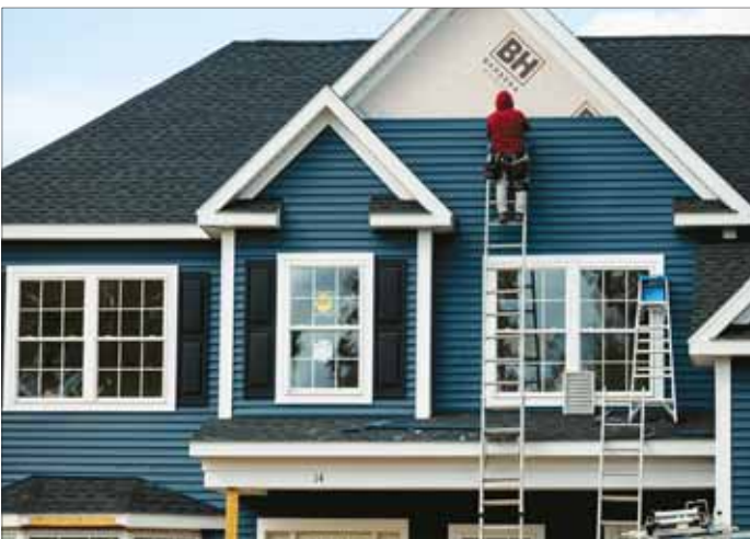
A worker installs siding on a home under construction at the Cold Spring Barbera Homes subdivision in Loudonville, New York. US single-family home-building surged to a five-month high in September, but permits for future construction rose only marginally amid excess supply of new homes on the market and prospective buyers holding out for lower mortgage rates.
