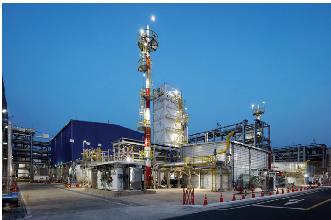
The world's largest sized liquid hydrogen production plant in Incheon Invested by SK E&S (operation started in May 2024).
