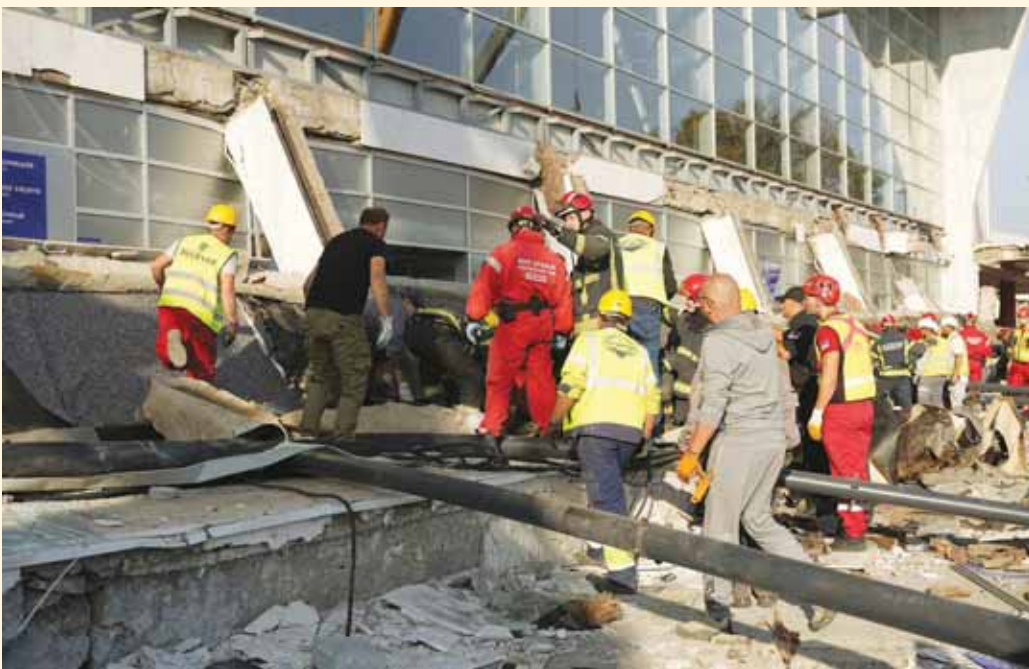
Rescue workers remove debris after a roof collapsed at the entrance to a railway station in Novi Sad, Serbia, yesterday.
