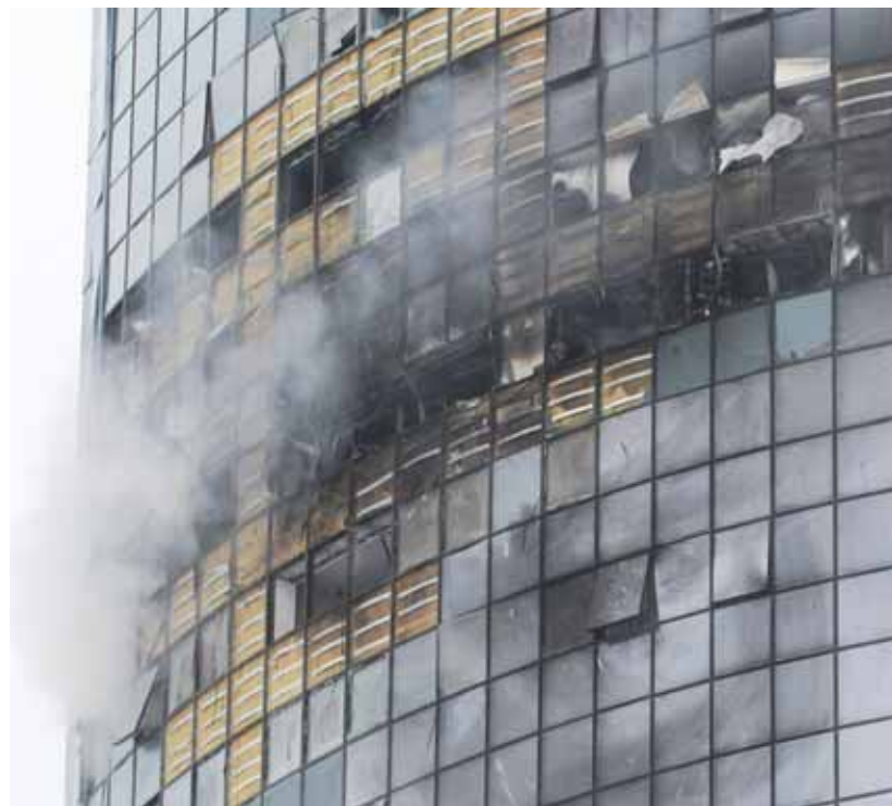
A view shows a damaged multi-storey residential building in Kazan following an alleged Ukrainian drone attack in the course of Russia-Ukraine conflict. (Reuters)
