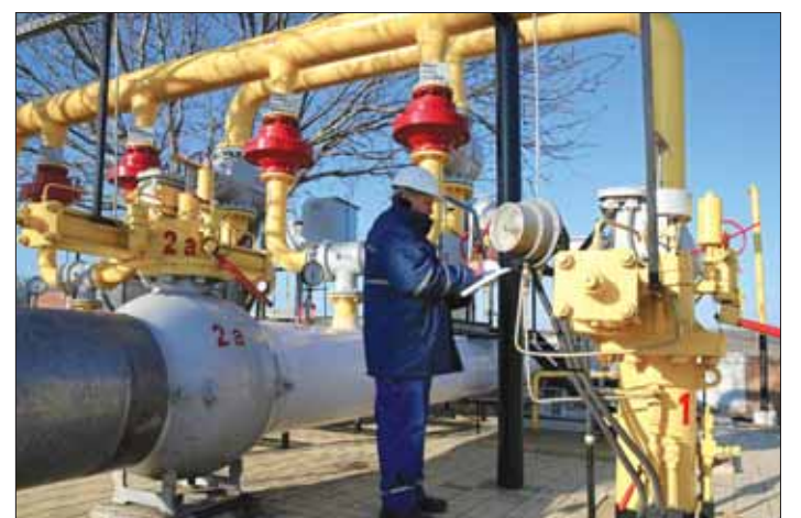
An employee works at the Chisinau-1 gas distribution plant of Moldovatransgaz energy company in Chisinau, Moldova, last March. (Reuters)
