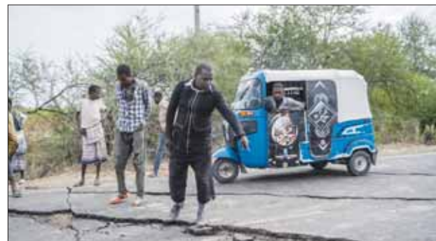
Residents assess the damage to a road affected by multiple earthquakes near the town of Kabanna, yesterday.
