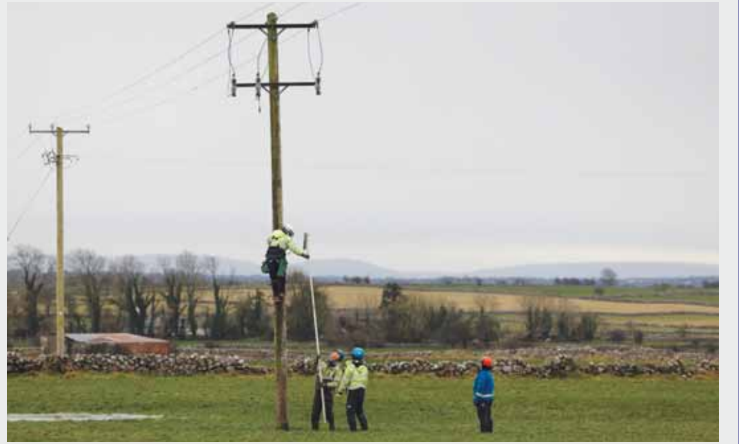
Electricians work to repair power lines in the aftermath of Storm Eowyn, in Currandrum, Ireland.
