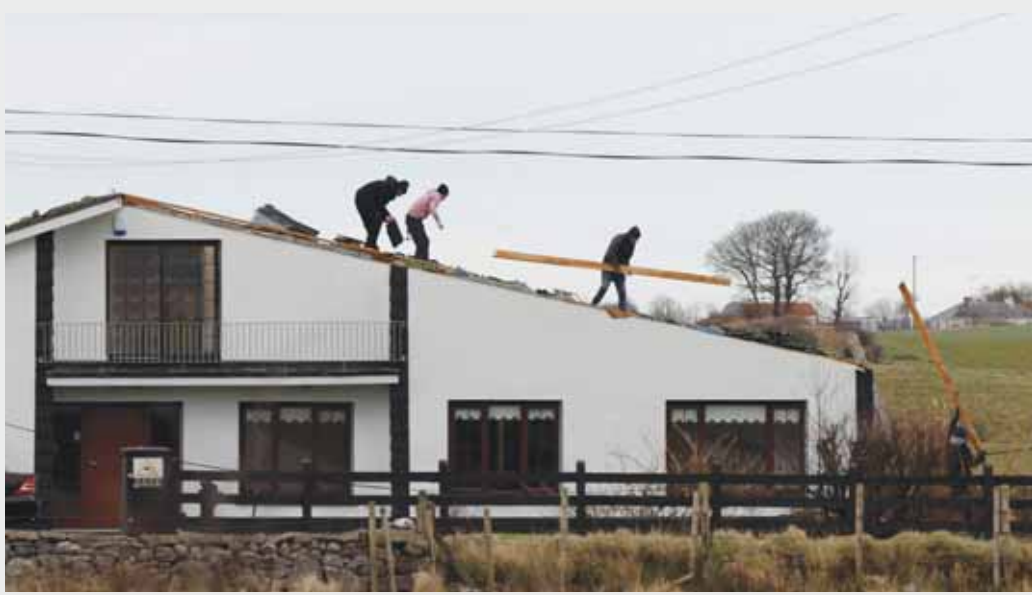
People work to repair the roof of their home in the aftermath of Storm Eowyn, in Tullinadaly, Ireland.
